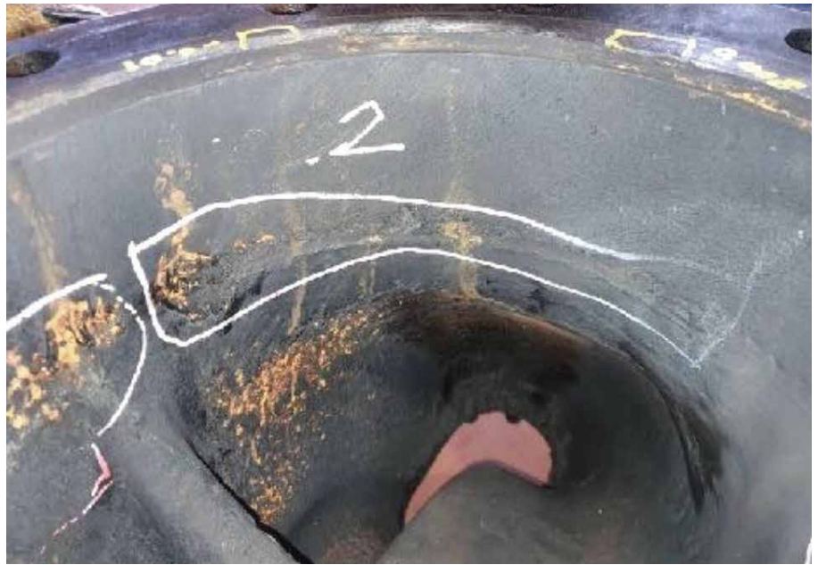
Fig. 3: Part of the eroded areas in the gas outlet nozzle (© DSI-Thailand)
